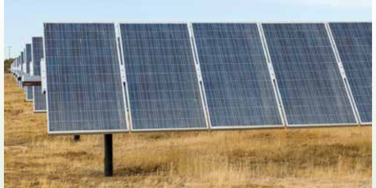
Solar panel array at Edwards Air Force Base, California. An Air Force photo by Giancarlo Casem
